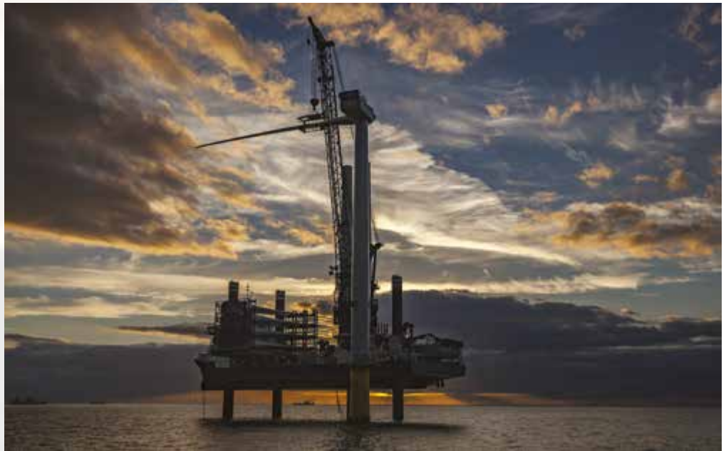
DONG Energy has invested around £6 billion in the UK since 2004, and will invest a further £6 billion in the Humber region by 2020. Photo courtesy of DONG Energy ©
